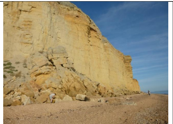
Landslip of fullers earth and underlying inferior oolite
